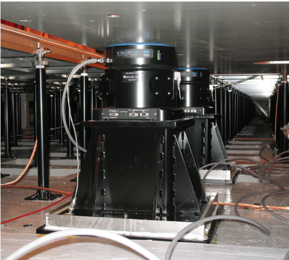
STACIS® 2100 on a “riser” installed under a TMC platform in a 36” tall raised floor
